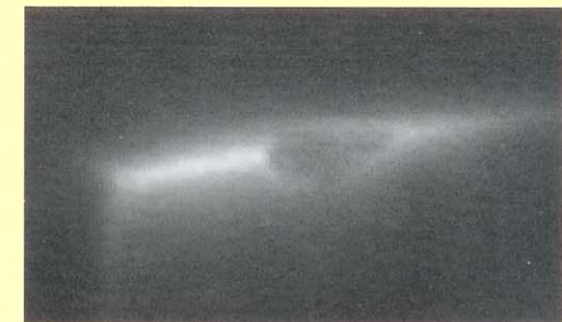
Photograph of live termite nest in wall as seen with the Thermal Imager.
